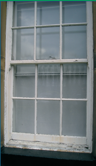
Window affected by wood decay.
