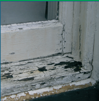
Wood decay at joints and cill require replacement.
